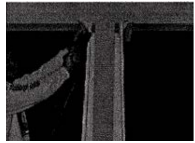
12. Raise cap to beam/soffit, center, and attach. There should be \frac{1}{4} " between column and cap platform.
