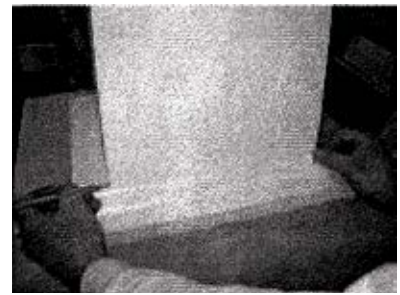
18. Use column shaft to mark cut lines for miters (cut long and work your way shorter for best results.)
