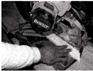
17. Using miter saw, cut base trim pieces to fit around bottom of column.
