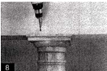
8. Pre-drill and countersink holes at an angle through the soffit into the capital. Secure with rust resistant screws.
